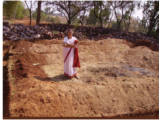
work at starting foundation level Inside Smt Saraswati Munenni fonder of Ashram and treasurer of society
